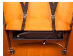
Battery underneath the bench
